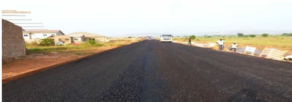
Construction of Western Bypass at Kasoa: Old Barrier to Kokrobite to Tuba to Sapato
